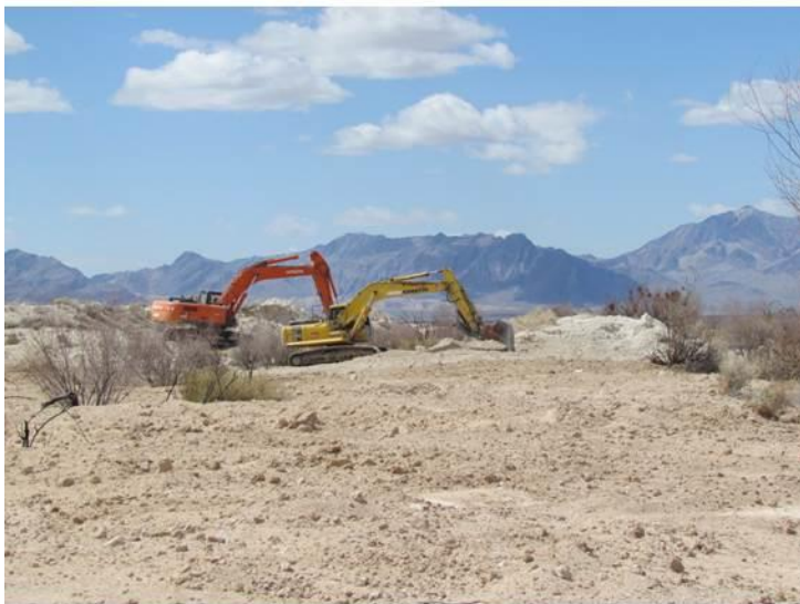
Figure 11. Berm and ditch removal in the Upper Carson Slough, Ash Meadows National Wildlife Refuge, NV. Photo courtesy of Hal Fairfield, volunteer.
