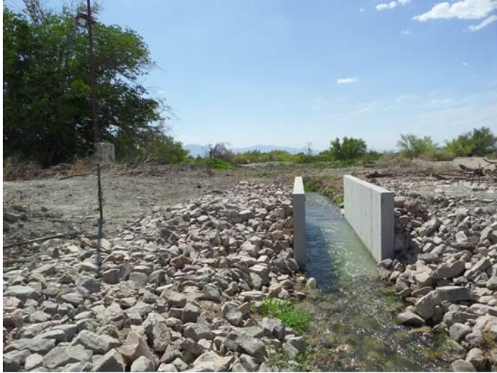
Figure 10. Concrete structure installed for water monitoring, Longstreet Spring, Ash Meadows National Wildlife Refuge, NV.
